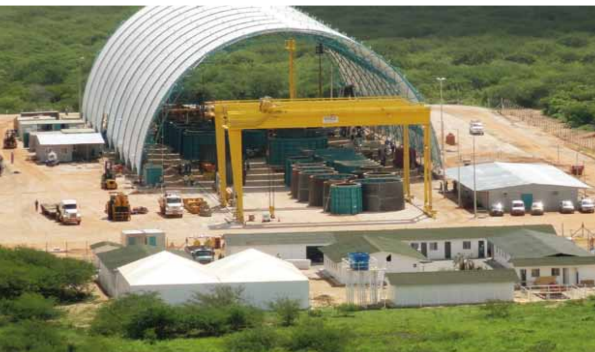
Light construction – ENERCON's mobile tower factory can be removed within few days.
