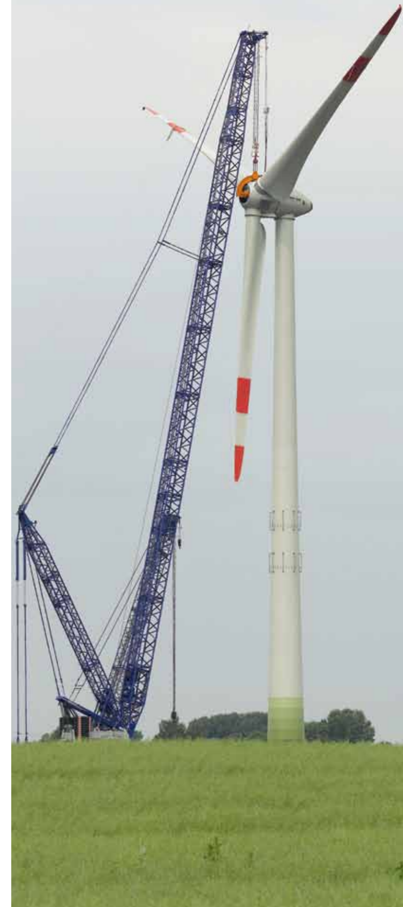
E-101 prototype installed.
